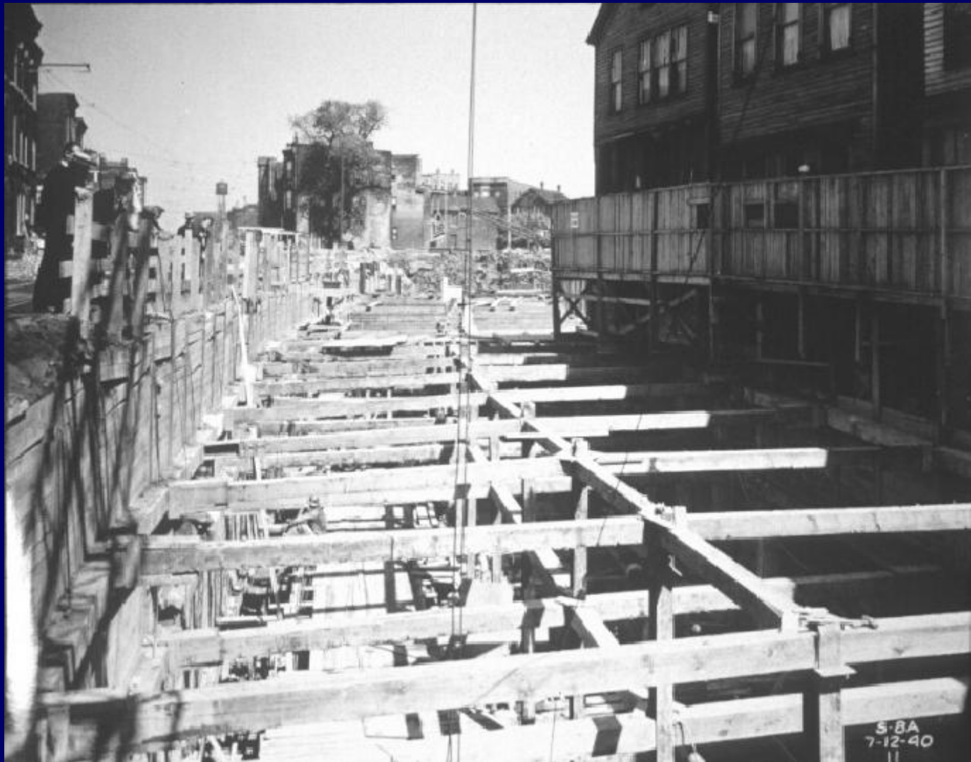
Braced open cut on Contract S-1A of the Chicago Subway This view shows the transition between the elevated and below ground sections of the State Street line, towards its north end, near the intersection with Clybourn Ave. In July 1940
